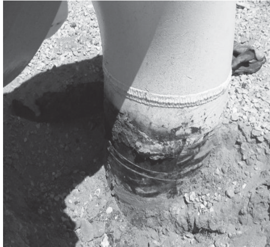
FIGURE 1. Corroded pipe due to accumulated soil and outside air
